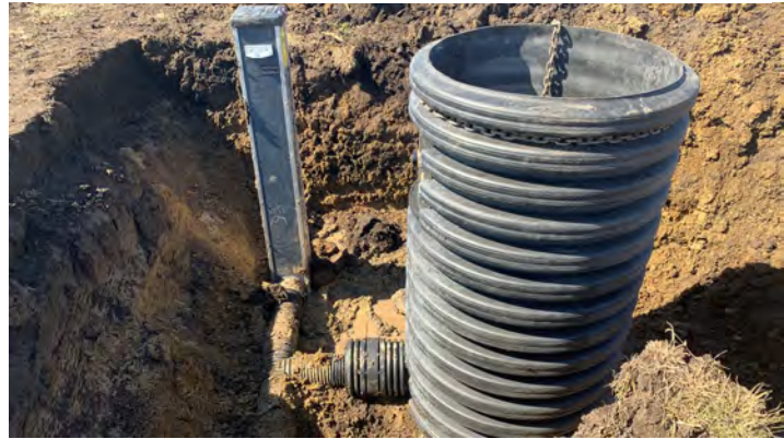
Figure 3. Gate Structures to Control Water Table
