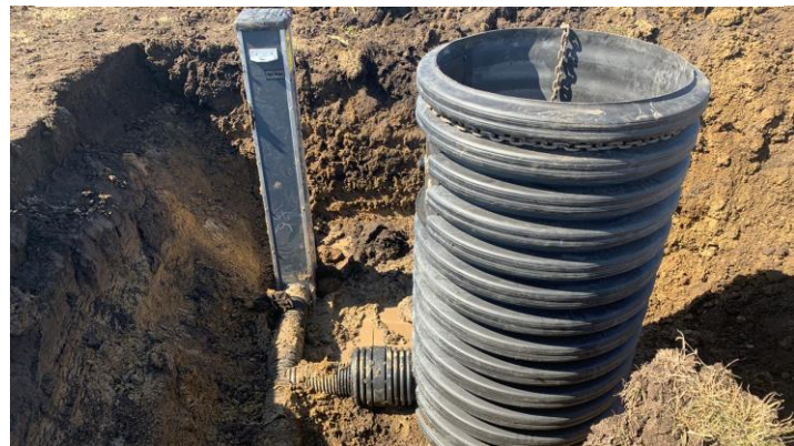
Figure 3. Gate Structures to Control Water Table
